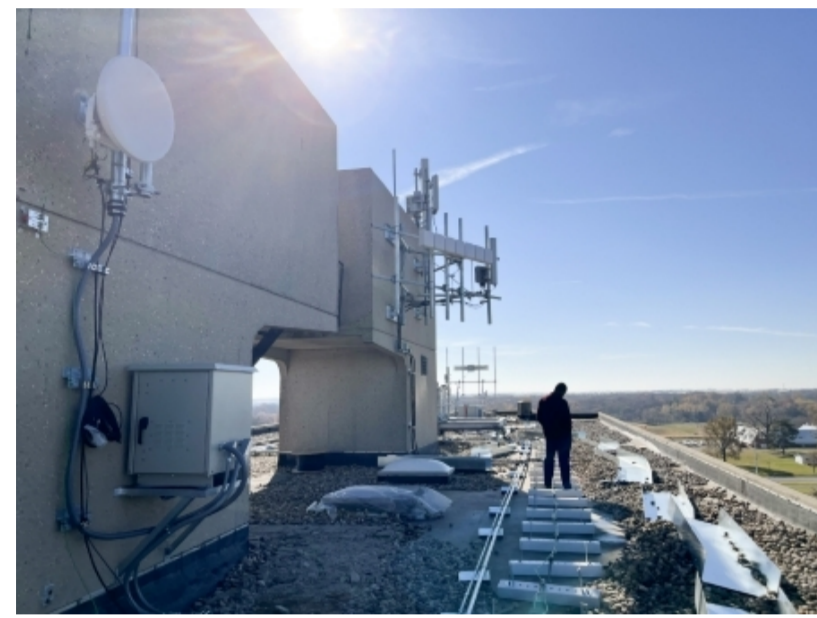
Figure 1. 5G radio infrastructure.
